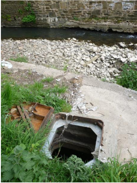
Missing manhole downstream of Briggate, by Robert Hellowell (1 of 3!)
