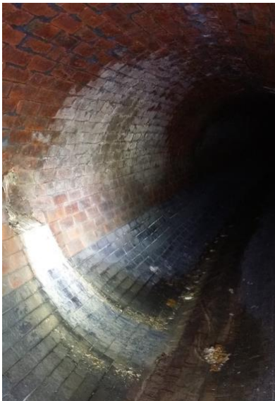
Outfall from Holiday Inn Premier Inn to Eastbrook with clear signs of pollution
